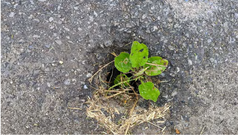
Figure F-4a Close-up of typical deck drain condition. Note, partial blockage from vegetation accumulation and growth.
