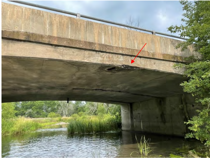
Figure F-10a General overview of north span fascia and outer parapet wall facing west. Note spall adjacent to deck drain missing outlet pipe.
