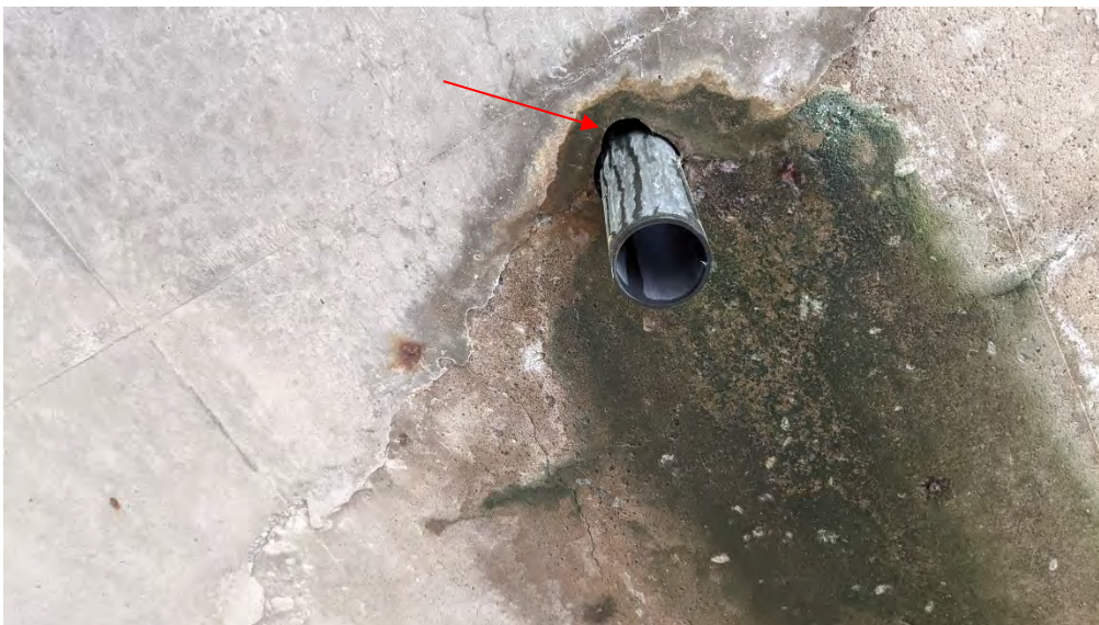
Figure F-4b Overview of typical condition of deck drain outlet. Note void around pipe and wet soffit.
