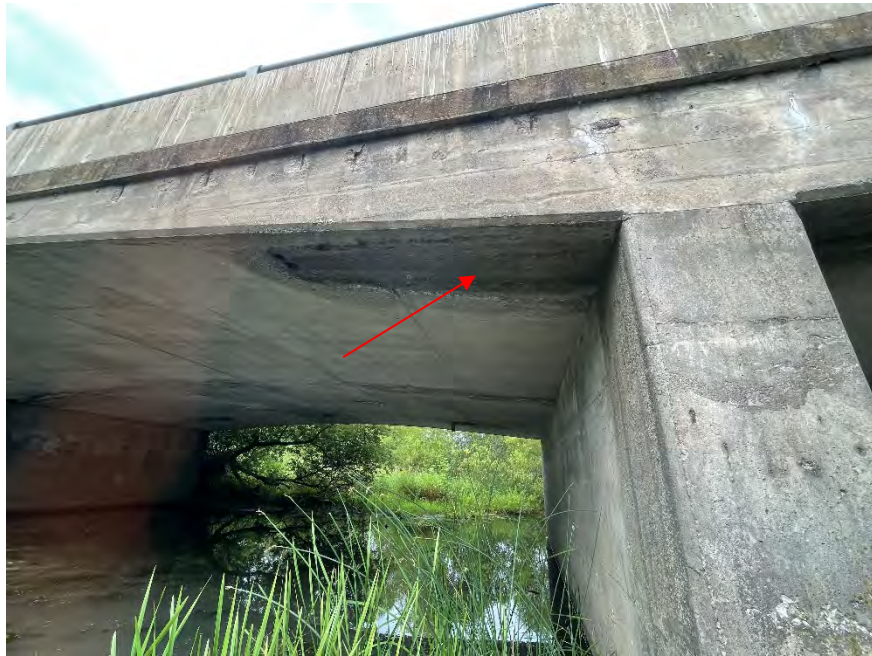
Figure F-11a Overview of bisecting pier interface with south span soffit facing west. Note missing outlet of deck drain wetting soffit and pier
