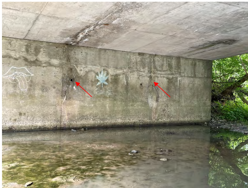
Figure F-9b Close up of south abutment facing south. Note vertical cracking.
