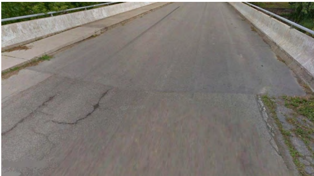
Figure F-3b Overview of paved over joint at south abutment facing north.
