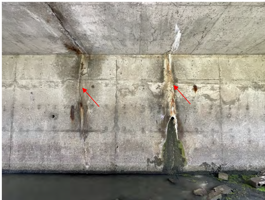
Figure F-8b Close up view of typical distresses observed on north abutment wall, note effloresce staining and reflective crack from centre span of soffit.
