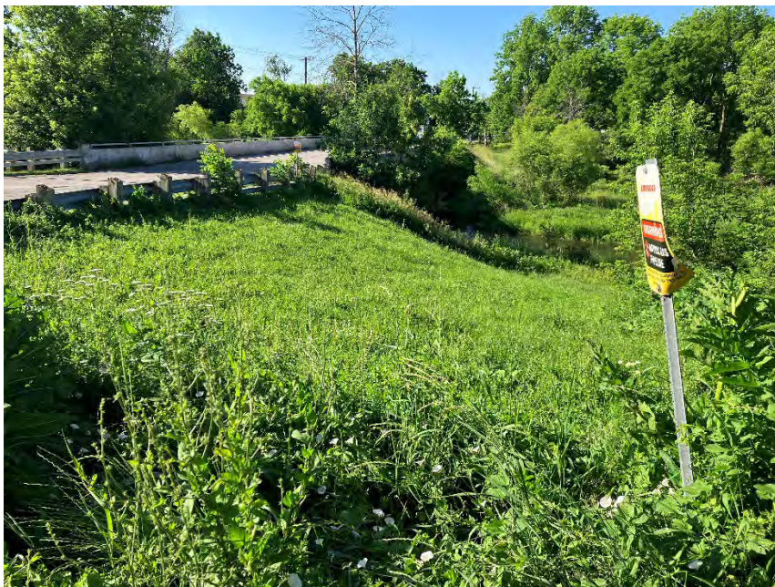
PHOTOGRAPH 2: View facing southeast of the study area from northwest of the bridge carrying St. Ann's Road across Twenty Mile Creek. Note the gas line signage in the foreground and steep slopes to Twenty Mile Creek.
