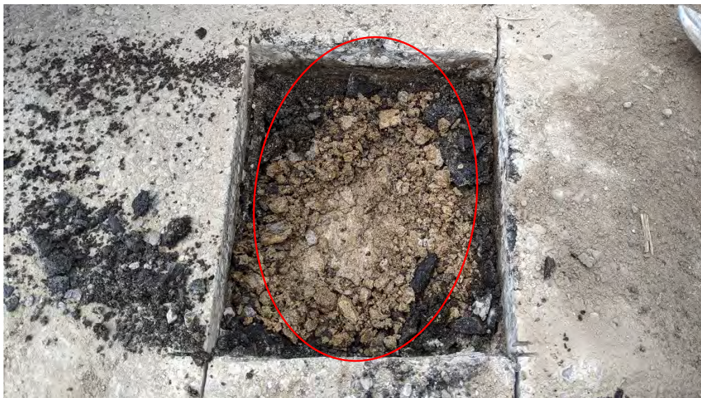
Figure F-7b Typical condition of concrete deck upon removal of asphalt from sawn samples. Note orange staining and disintegrated concrete to a depth approximately 50 mm.
