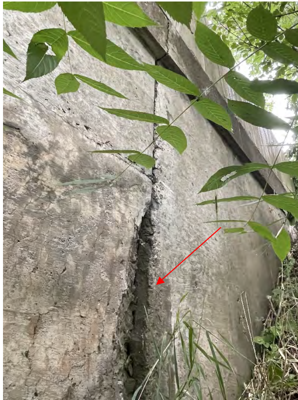
Figure F-13a General overview of northeast wing wall facing west. Note severe spall at construction joint.
