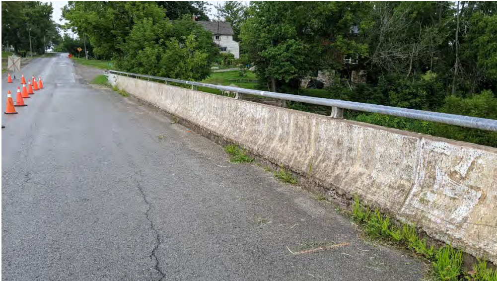
Figure F-6b Typical condition of east parapet wall and guardrail facing north.
