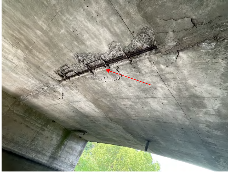
Figure F-12a General overview of north span soffit facing east, note severe spall with severely corroded rebar along centre of soffit.
