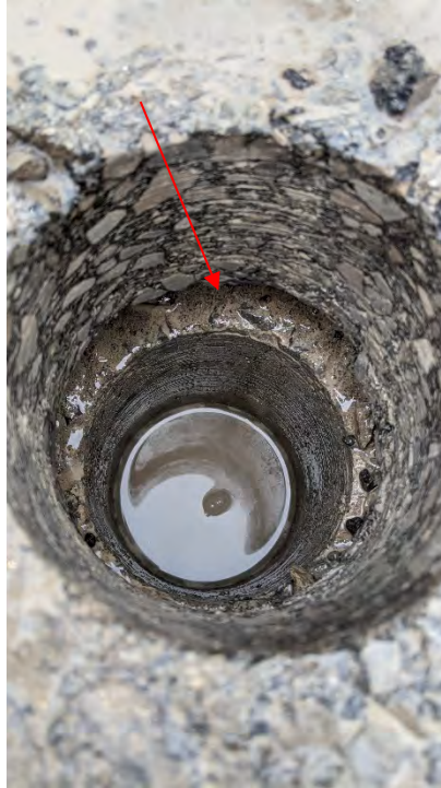
Figure F-7a Typical condition of concrete deck during core extraction. Note void below asphalt at concrete deck interface due to deterioration of concrete surface to a depth of approximately 50 mm.
