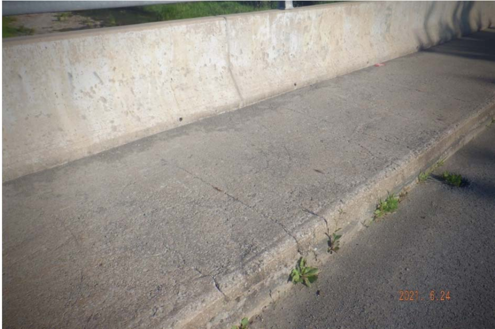
Photo No. 3: Deterioration of sidewalk on west side of road (typical).
