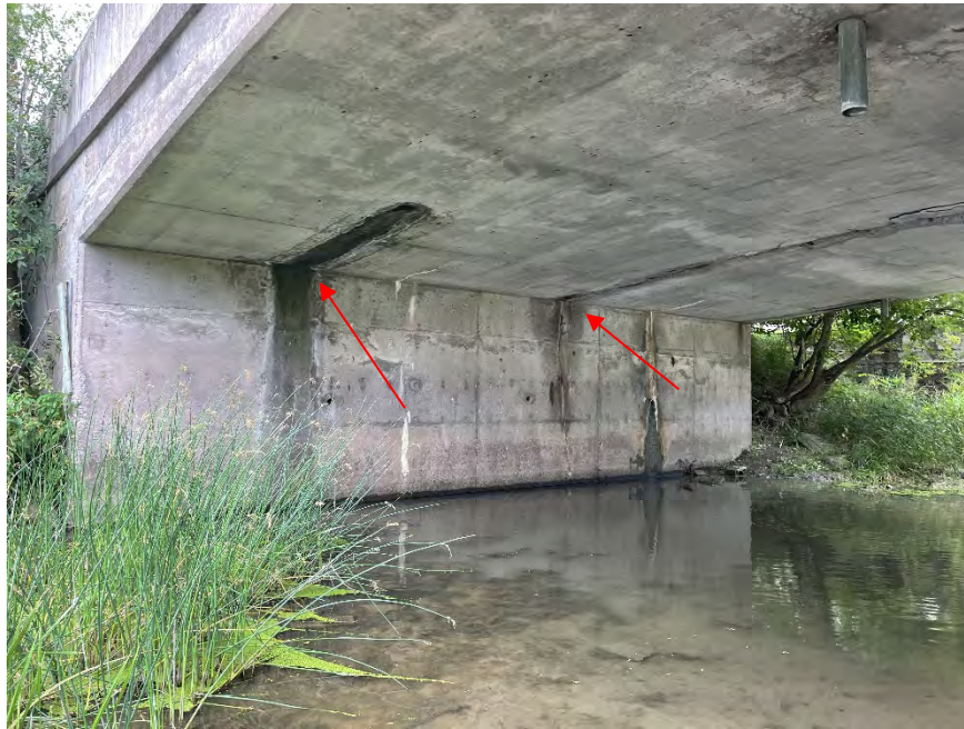
Figure F-8a Overview of north abutment facing northeast. Note northwest deck drain missing outlet pipe section and wetting soffit/abutment wall. Note wide crack down centre of soffit wetting abutment wall.
