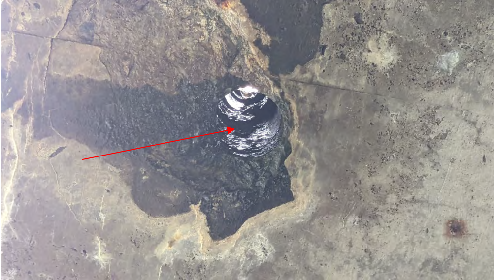
Figure F-5a Close up of east deck drain at station 23.5 metres. Note outlet pipe is completely corroded and pipe embedded in concrete deck is completely corroded with severe scaling.
