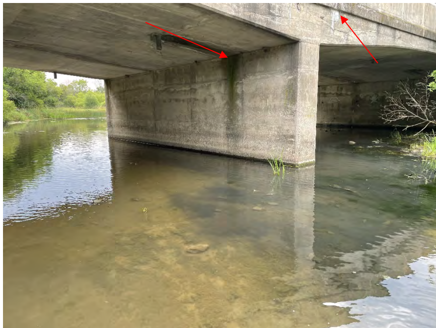
Figure F-11b General overview of bisecting pier and north span interface facing southeast. Note deck drain wetting soffit and pier.
