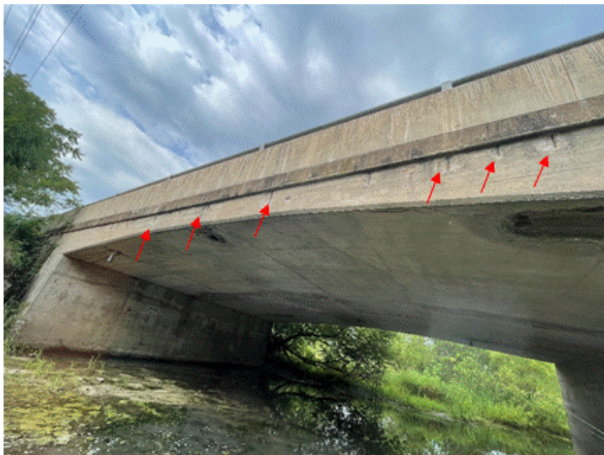
Figure F-10b General overview of south span fascia and outer parapet wall facing west. Note localized spalling with exposed moderately corroded rebar.
